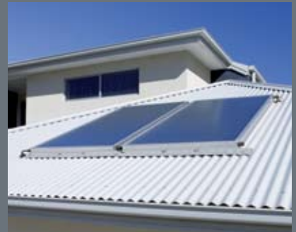
Gas Boosted Solar Hot Water
